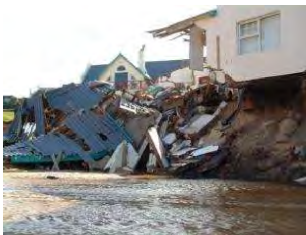
(c) Flood damage
